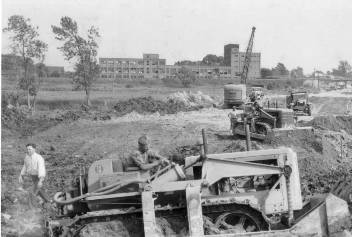
1939 Route 1 Bypass construction, rear of Morley Factory Paper Buildings (#11, 11a, 11b), facing east (Collection of Portsmouth Athenaeum)
